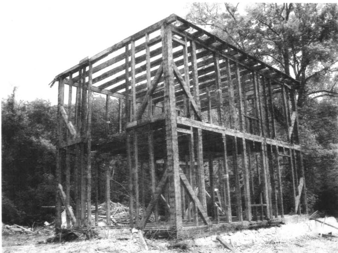
THIS TIMBER FRAME SKELETON RESEMBLES PRETTY MUCH HOW THE BANKS BUILDING'S FRAME APPEARED WHEN IT WAS BEING BUILT. BRACES WERE AT THE TOP OF THE POST NOT AT THE BOTTOM.
