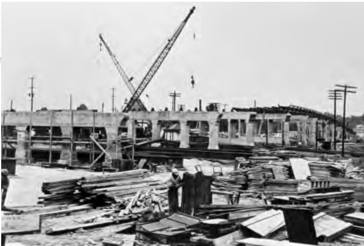
Construction of the Elsmere Viaduct over the B&O Railroad in 1948. The bridge eliminated a dangerous railroad crossing and was an early example of a continuous-span steel multi girder bridge designed by the state highway department's bridge division.
