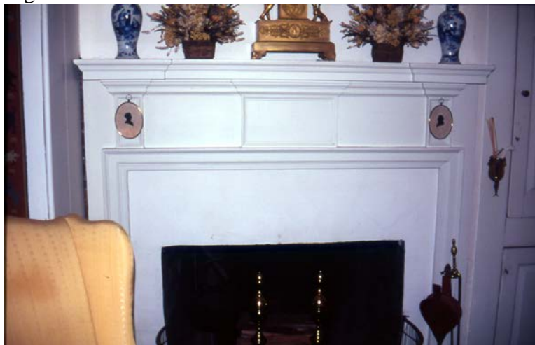
Fig. 9. First floor front room mantelpiece. Note the narrow gap with the exposed bricks to its left.
